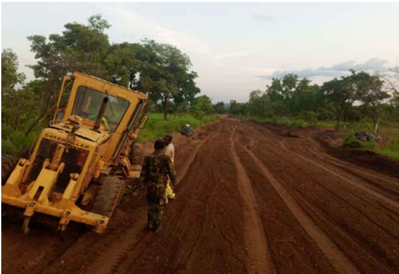
Figure 2:12: Construction Works of the Feeder Road at Sapelliga facilitated by the Ghana Boundary Commission.
